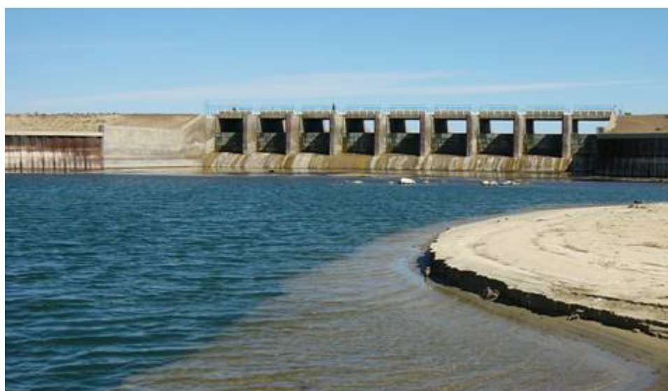
Completed dike and water spillway view from tailrace, September 23, 2007 (Photo by I. Plotnikov)
